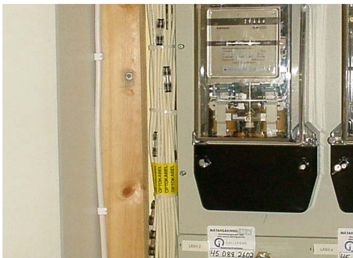
Figure 4: Microduct bundles with splices in a cabinet for electricity metering equipment
