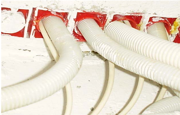
Figure 5: Pass way for micro ducts in electricity riser
