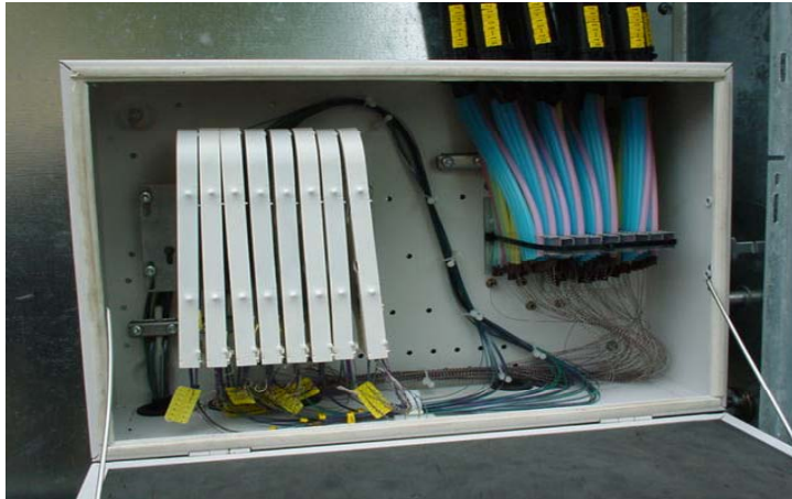
Figure 7: Interior arrangement with splice cabinet inside street cabinet
