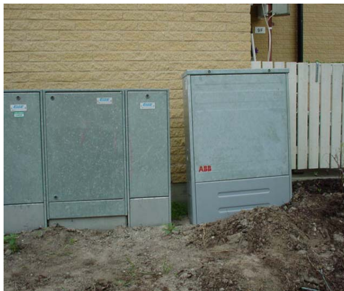
Figure 6: Outdoor splice cabinet to the right
