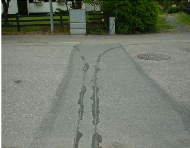
Figure 5: Fiber grooves on the pavement
