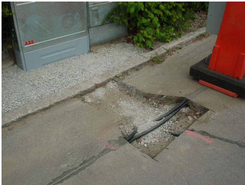
Figure 6 : Microduct containing air blown fiber
